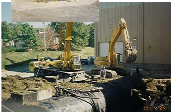
Photos (top to bottom): Geoprobe 5400 in use; Western Illinois University Underground Storage Tank removal and above ground replacement (completed and during construction).
